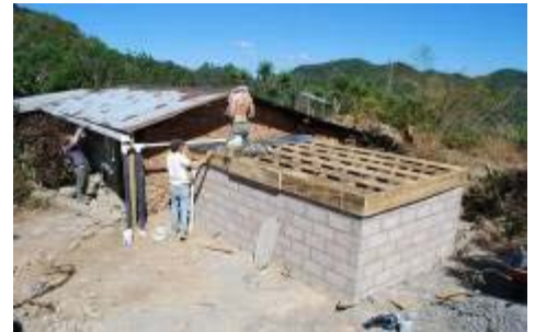
View of the rainwater catchment tank as the roof is being constructed.
