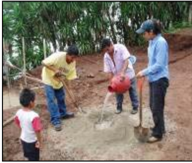
An EWB-OSU member works with beneficiaries to mix cement by the "volcano method."
