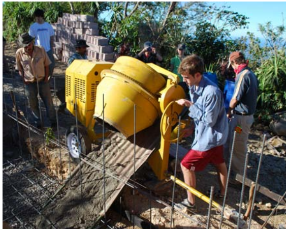
Pouring the foundation at the sub-community of Cerro Cabollo on the December 2008 Trip.
