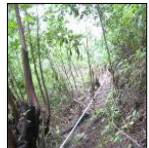
Galvanized pipe along the steep, forested hillside.
